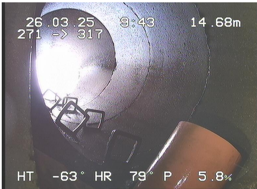
271-317_264.jpg, 00:01:26, 14.68m Endknoten, Rohrende, 317
