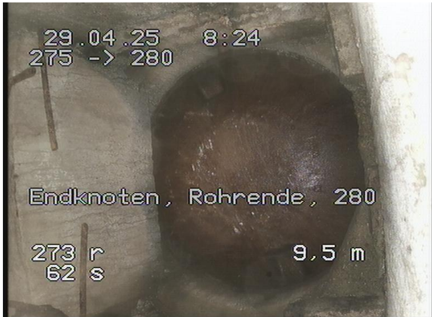
275-280_418.jpg, 00:05:50, 9.50m Endknoten, Rohrende, 280
