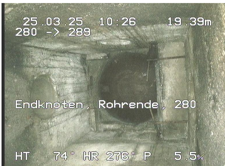
280-289_203.jpg, 00:01:39, 19.39m Endknoten, Rohrende, 280
