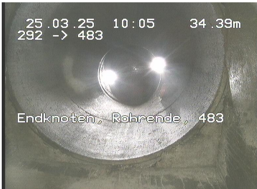
292-483_195.jpg, 00:02:52, 34.39m Endknoten, Rohrende, 483
