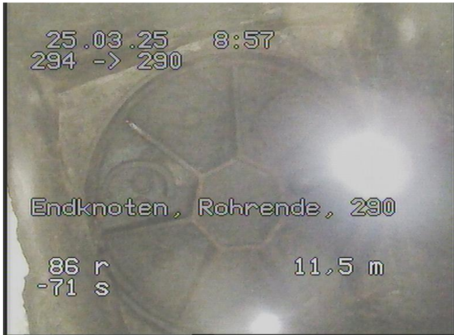
294-290_166.jpg, 00:01:20, 11.50m Endknoten, Rohrende, 290
