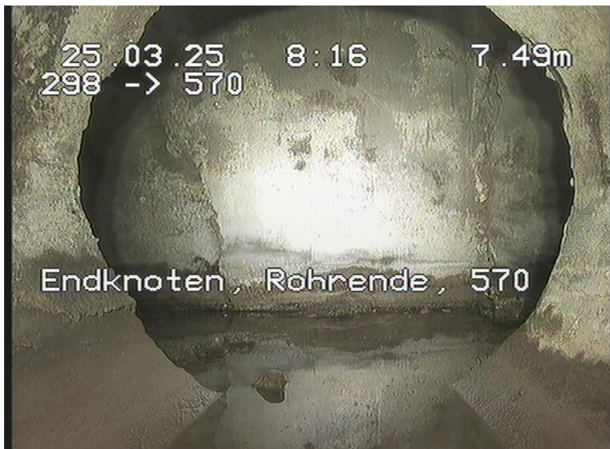
298-570_146.jpg, 00:01:31, 7.49m Endknoten, Rohrende, 570
