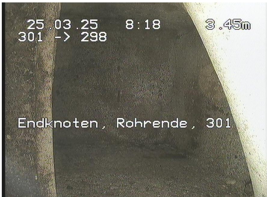
301-298_148.jpg, 00:01:10, 3.45m Endknoten, Rohrende, 301
