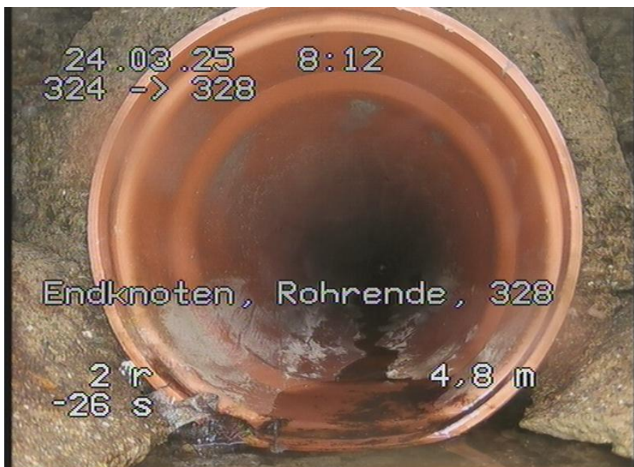
324-328_28.jpg, 00:00:41, 4.80m Endknoten, Rohrende, 328
