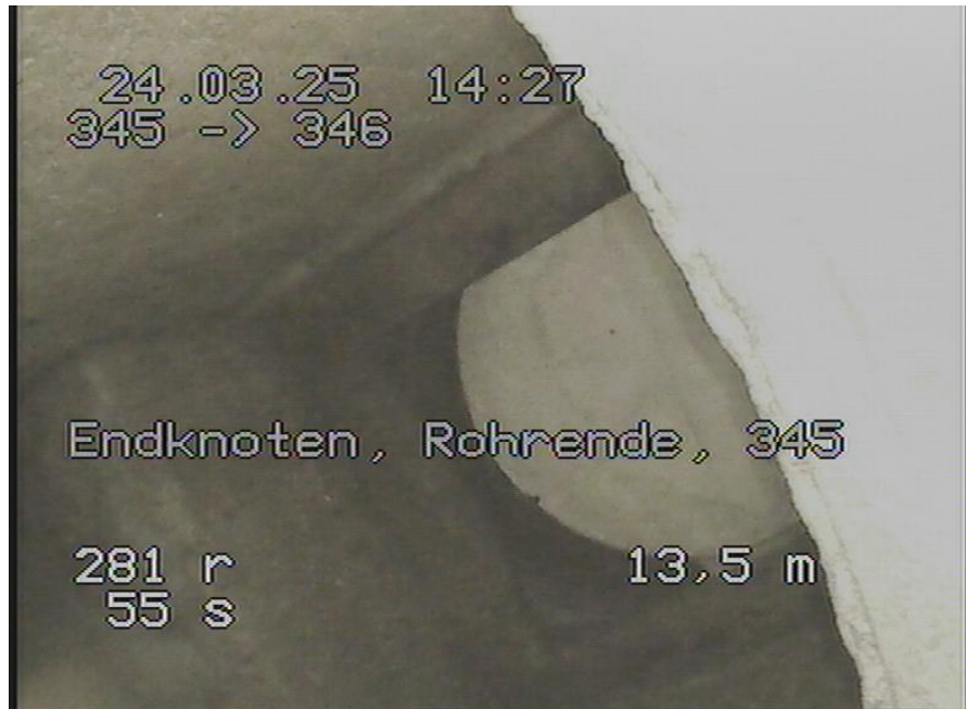
345-346_119.jpg, 00:02:25, 13.50m Endknoten, Rohrende, 345
