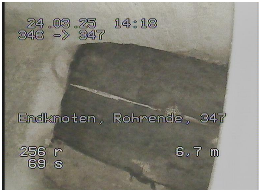
346-347_115.jpg, 00:01:12, 6.70m Endknoten, Rohrende, 347
