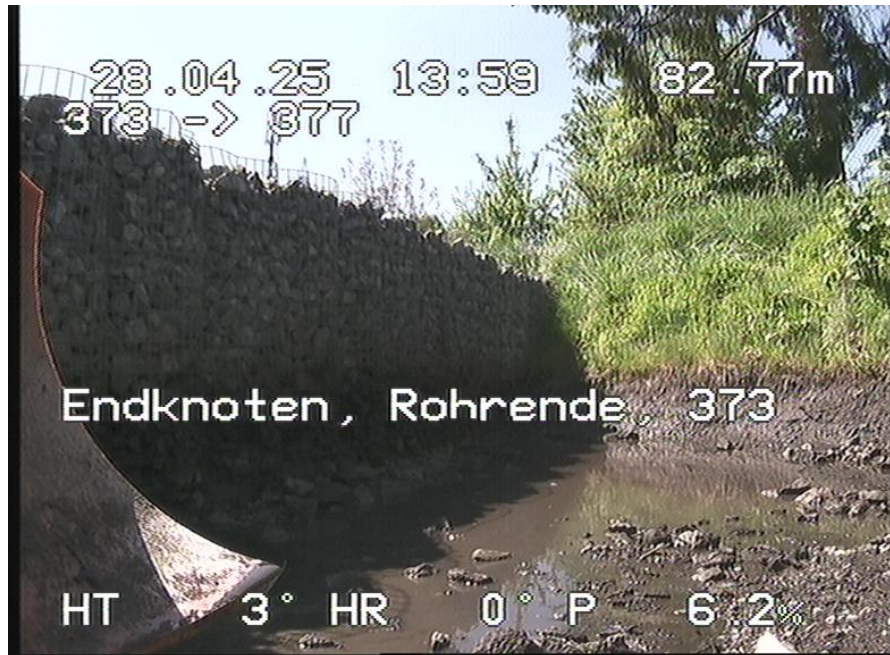
373-377_400.jpg, 00:05:43, 82.77m Endknoten, Rohrende, 373
