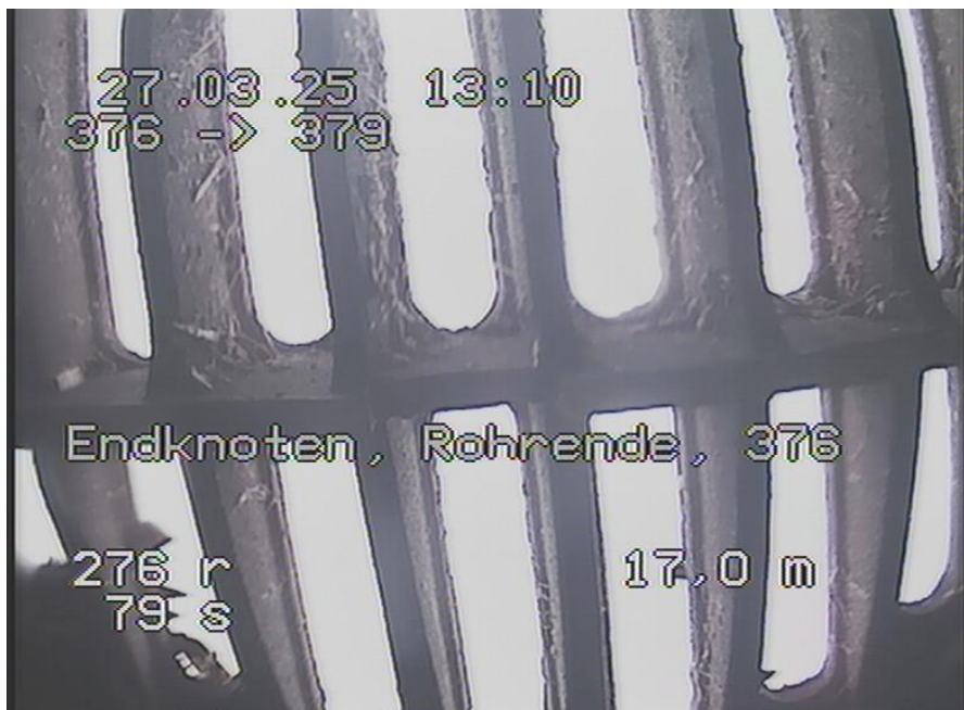
376-379_378.jpg, 00:00:52, 17.00m Endknoten, Rohrende, 376
