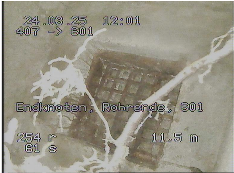
407-601_72.jpg, 00:02:49, 11.50m Endknoten, Rohrende, 601
