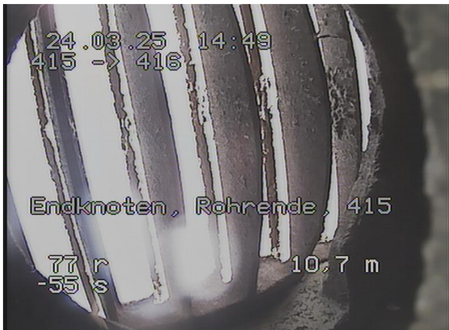
415-416_136.jpg, 00:00:37, 10.70m Endknoten, Rohrende, 415
