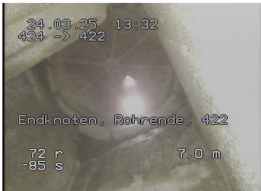
424-422_106.jpg, 00:00:55, 7.00m Endknoten, Rohrende, 422
