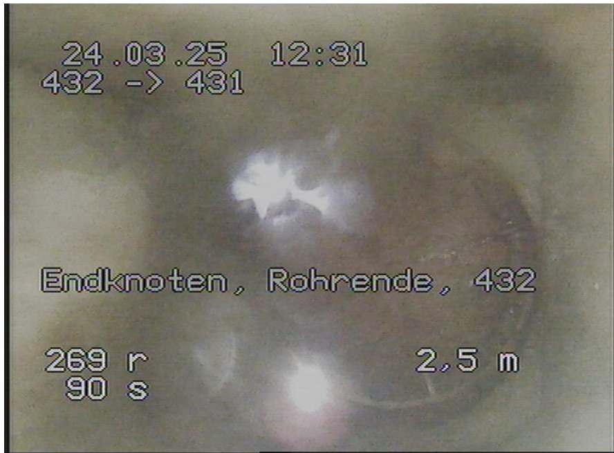
432-431_78.jpg, 00:00:39, 2.50m Endknoten, Rohrende, 432
