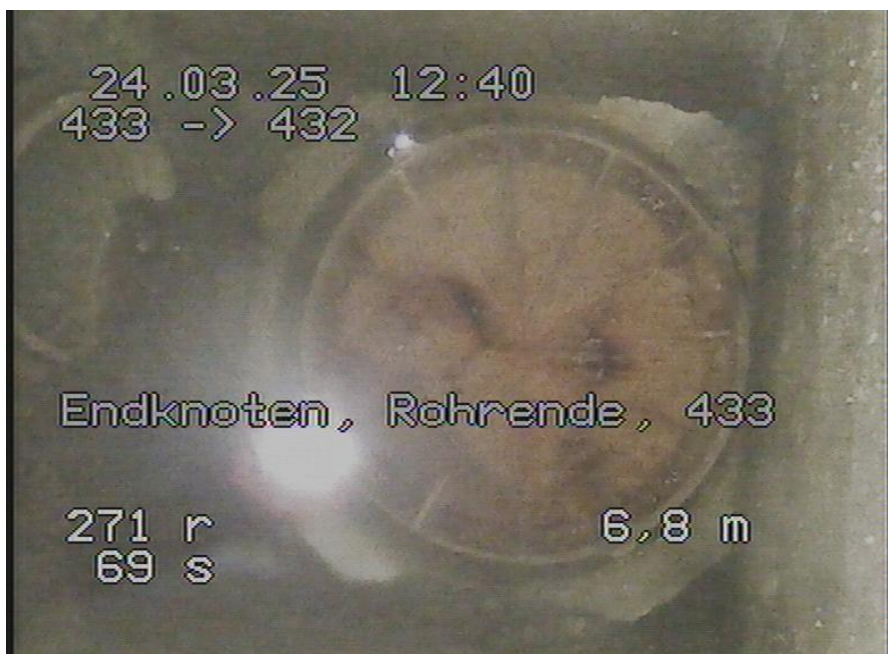
433-432_82.jpg, 00:00:42, 6.80m Endknoten, Rohrende, 433
