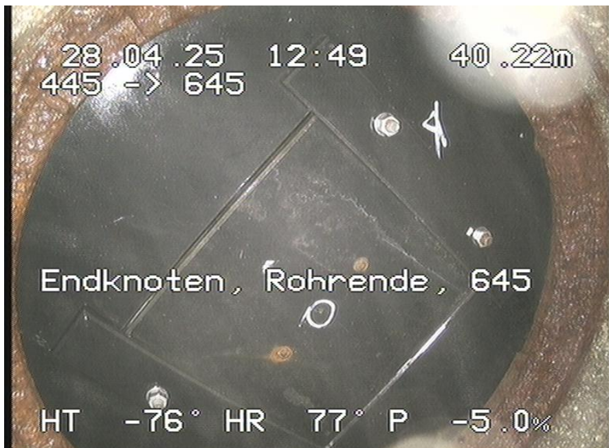
445-645_395.jpg, 00:02:38, 40.08m Endknoten, Rohrende, 645
