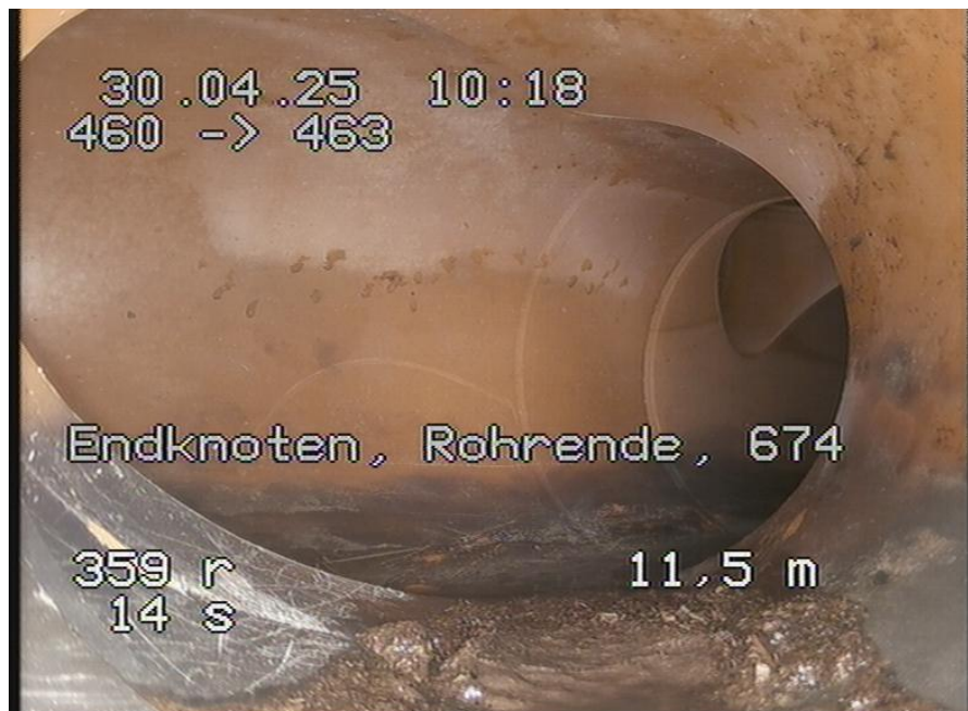
460-463_480.jpg, 00:01:22, 11.50m Endknoten, Rohrende, 674
