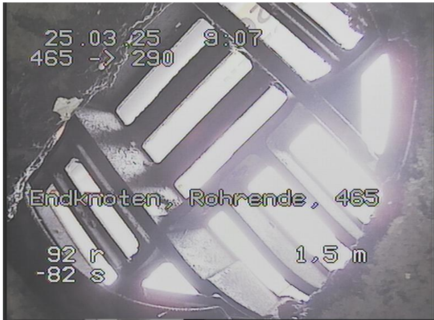
465-290_168.jpg, 00:00:31, 1.50m Endknoten, Rohrende, 465
