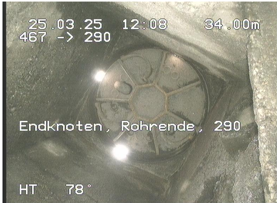
467-290_235.jpg, 00:01:15, 34.00m Endknoten, Rohrende, 290
