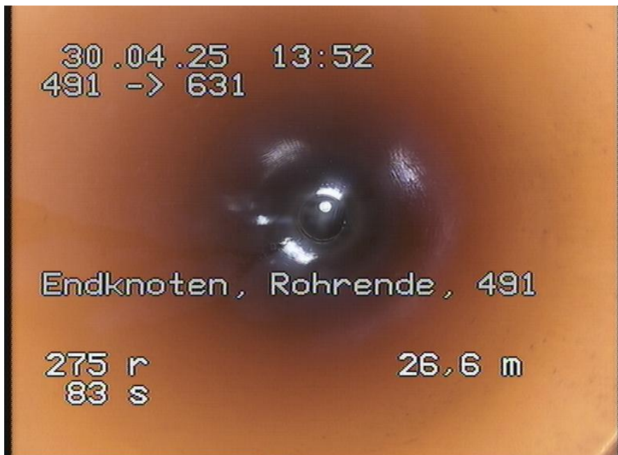
491-631_513.jpg, 00:02:46, 26.60m Endknoten, Rohrende, 491
