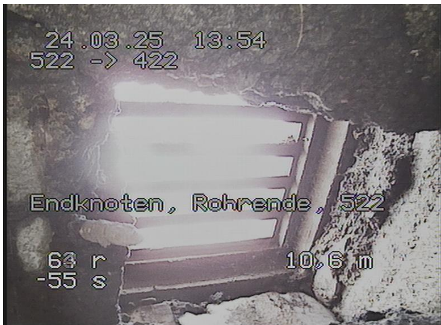
522-422_110.jpg, 00:01:07, 10.60m Endknoten, Rohrende, 522
