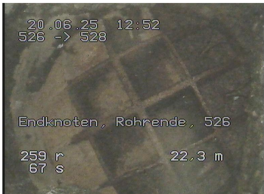
526-528_701.jpg, 00:01:03, 22.30m Endknoten, Rohrende, 526
