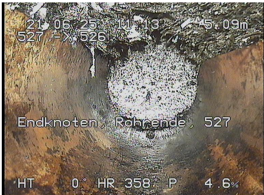
527-526_732.jpg, 00:02:11, 5.09m Endknoten, Rohrende, 527
