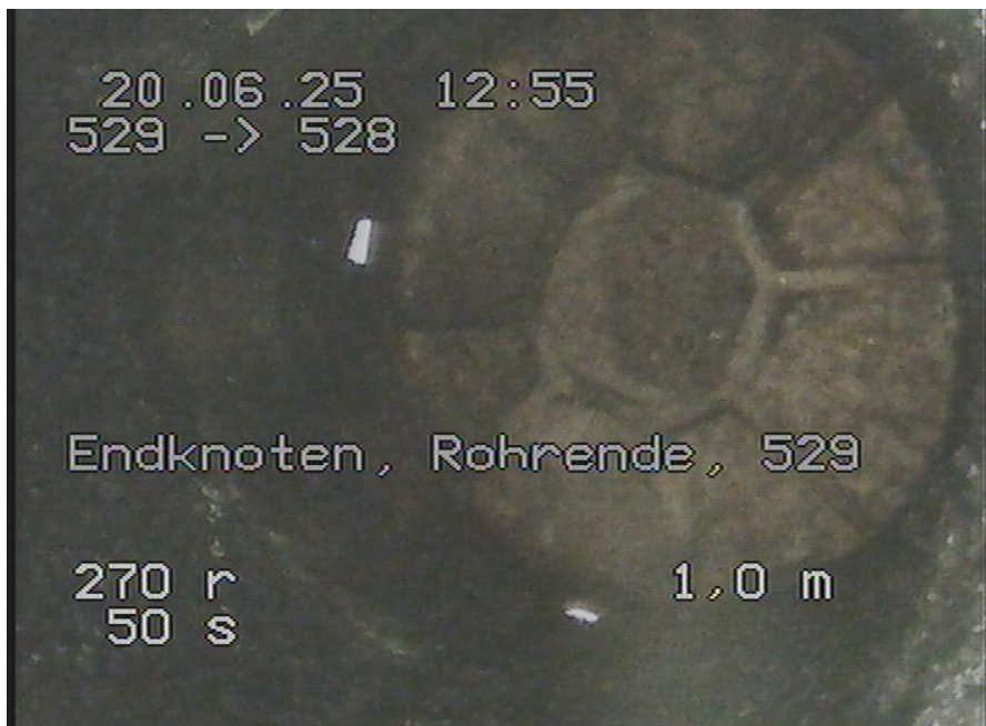
529-528_703.jpg, 00:00:14, 1.00m Endknoten, Rohrende, 529
