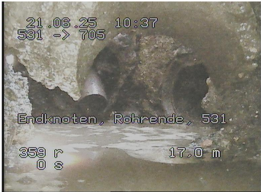
531-705_728.jpg, 00:02:50, 17.00m Endknoten, Rohrende, 531
