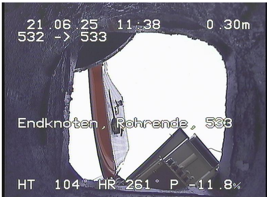
532-533_741.jpg, 00:00:24, 0.30m Endknoten, Rohrende, 533
