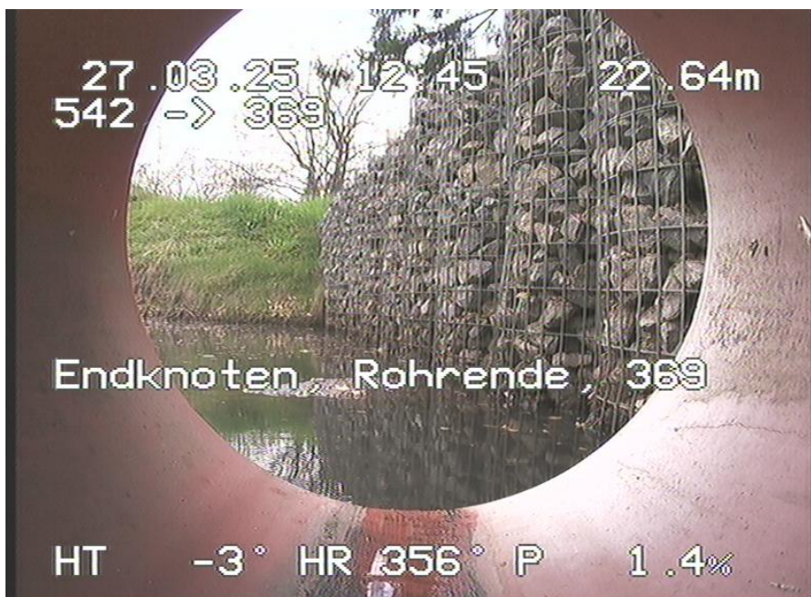
542-369_374.jpg, 00:02:00, 22.64m Endknoten, Rohrende, 369
