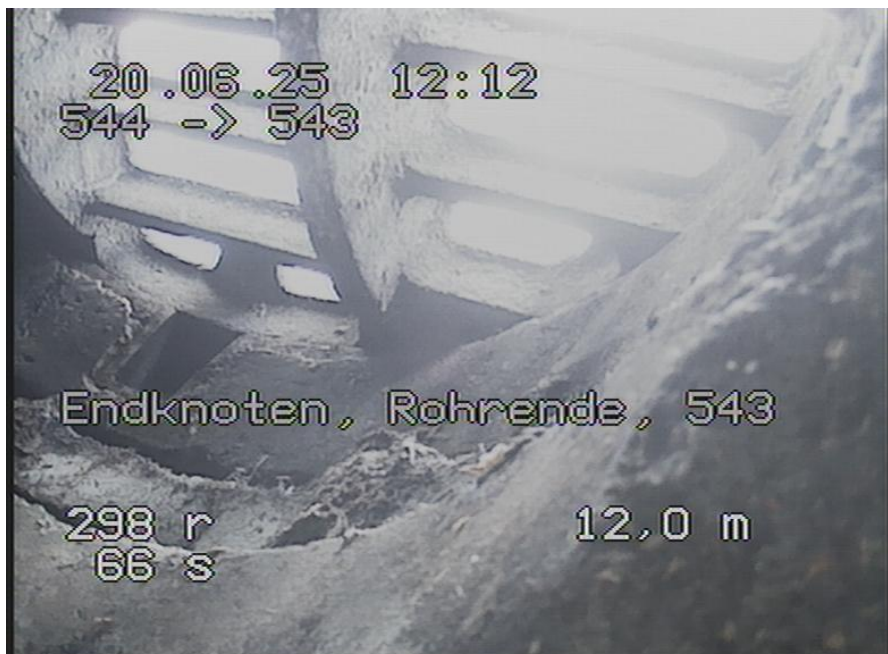
544-543_687.jpg, 00:00:53, 12.00m Endknoten, Rohrende, 543
