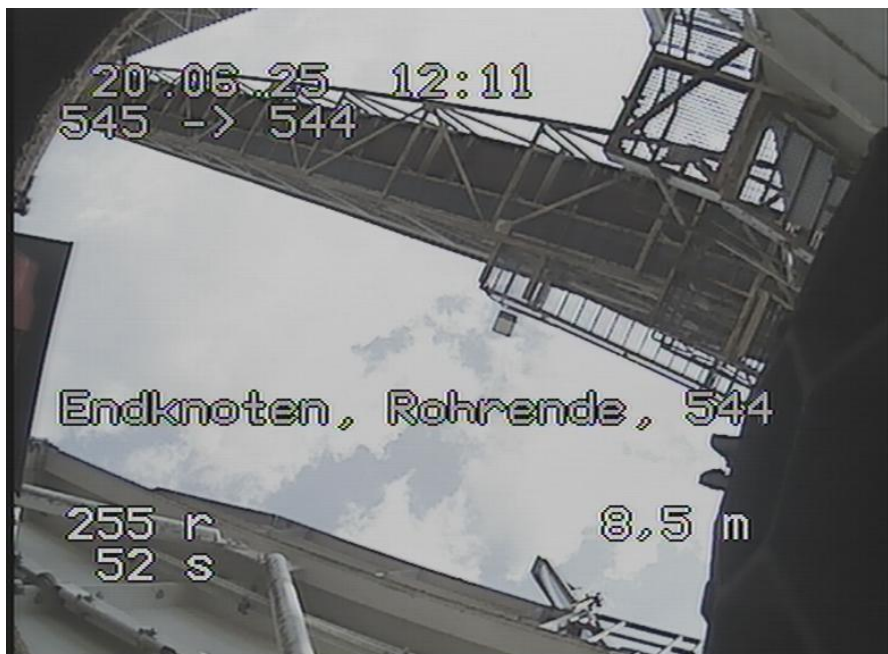
545-544_685.jpg, 00:00:32, 8.50m Endknoten, Rohrende, 544
