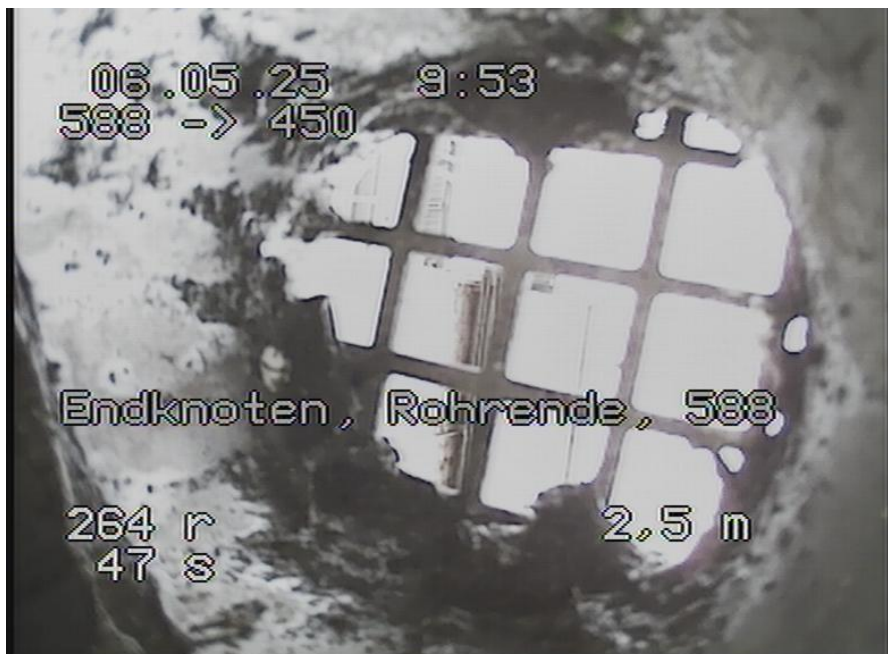
588-450_538.jpg, 00:01:15, 2.50m Endknoten, Rohrende, 588
