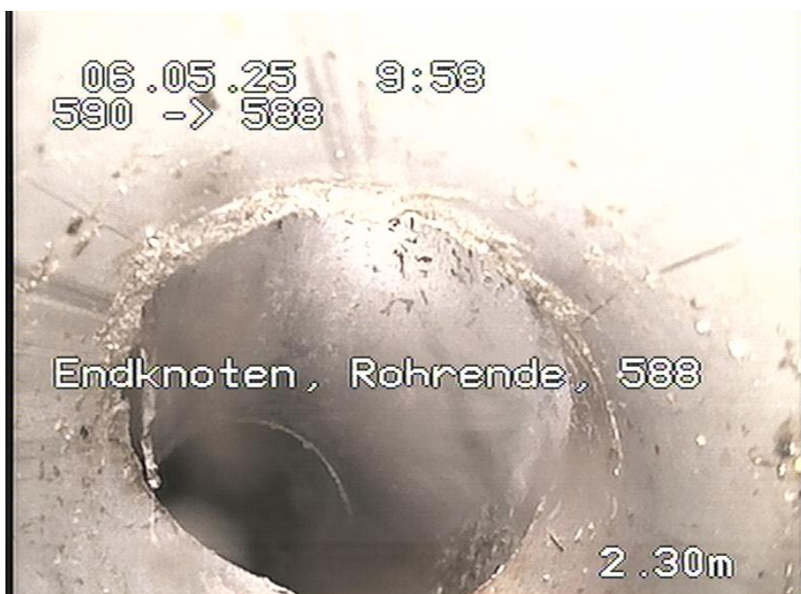
590-588_540.jpg, 00:00:49, 2.30m Endknoten, Rohrende, 588
