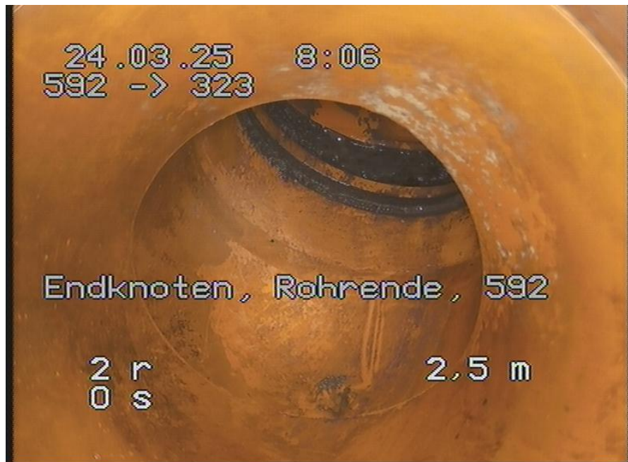
592-323_20.jpg, 00:00:54, 2.50m Endknoten, Rohrende, 592
