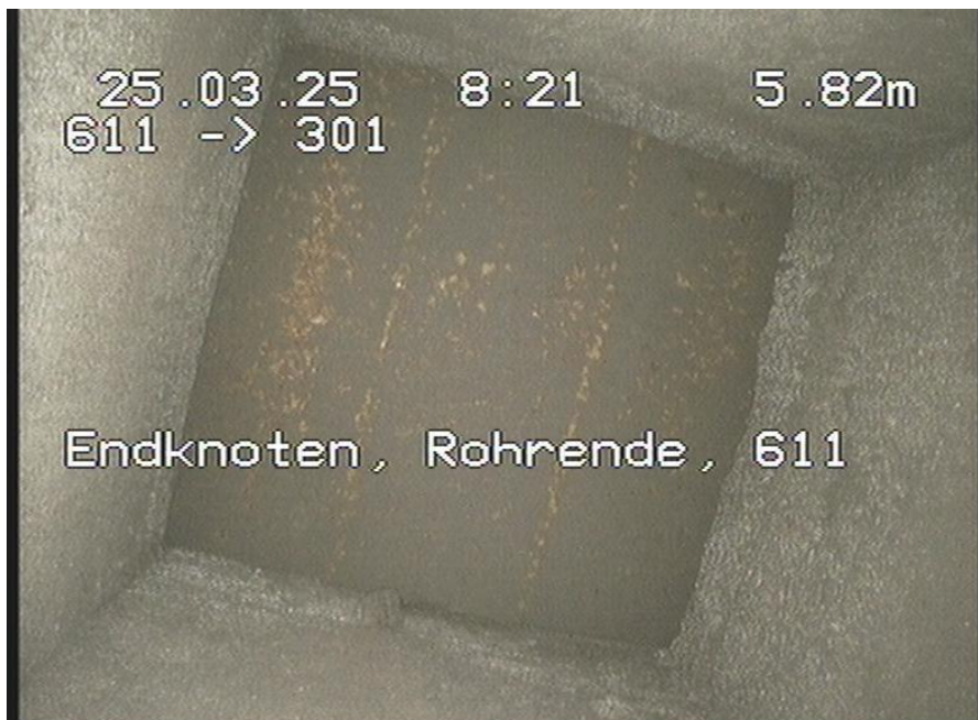
611-301_150.jpg, 00:00:58, 5.82m Endknoten, Rohrende, 611
