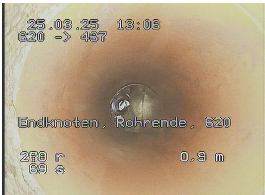
620-467_247.jpg, 00:00:19, 0.90m Endknoten, Rohrende, 620
