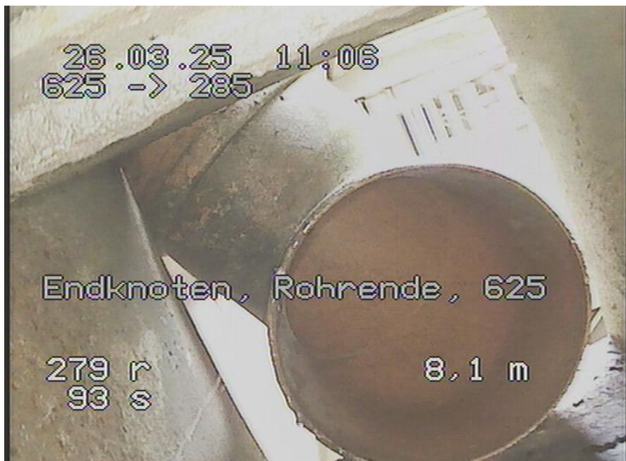
625-285_270.jpg, 00:01:43, 8.10m Endknoten, Rohrende, 625
