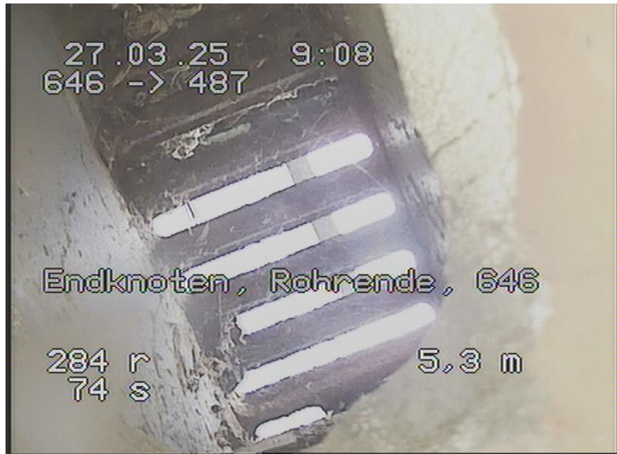
646-487_351.jpg, 00:01:14, 5.30m Endknoten, Rohrende, 646
