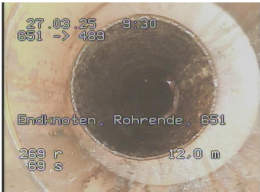
651-489_357.jpg, 00:01:25, 12.00m Endknoten, Rohrende, 651
