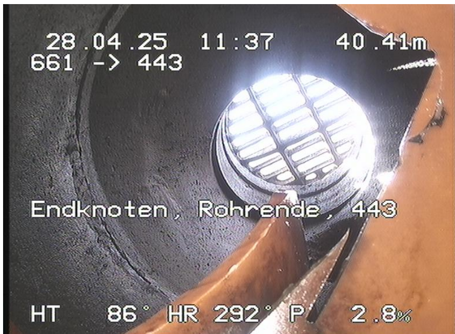
661-443_392.jpg, 00:03:05, 40.41m Endknoten, Rohrende, 443
