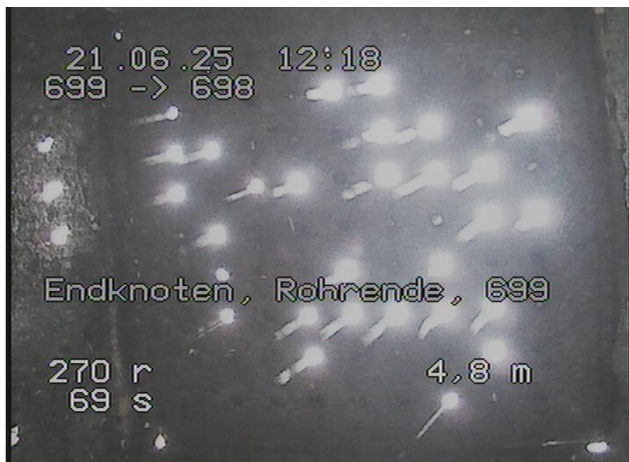
699-698_756.jpg, 00:00:28, 4.80m Endknoten, Rohrende, 699
