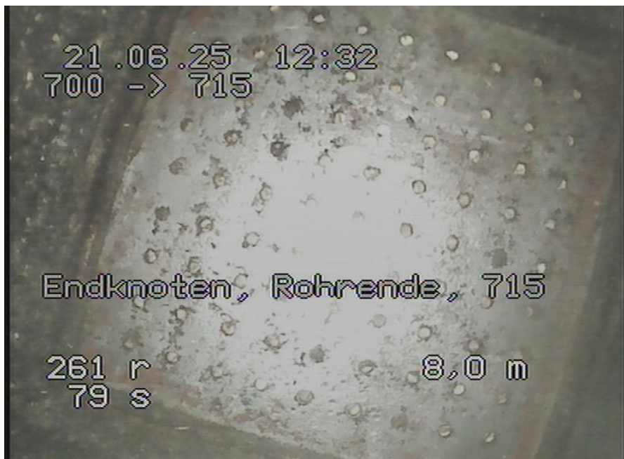
700-715_762.jpg, 00:00:39, 8.00m Endknoten, Rohrende, 715
